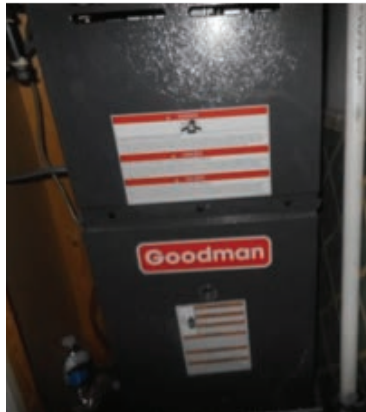
After – New Energy Efficient Heating System
