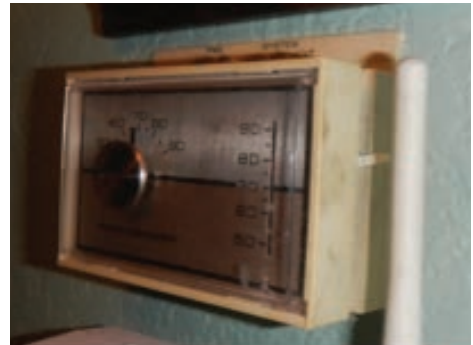
Before – Outdated manual thermostat
