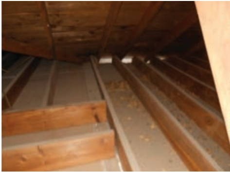
Before – Bare attic floor no protection from heat or cold.
