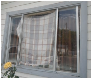
Before – Broken window let hot/cold air through
